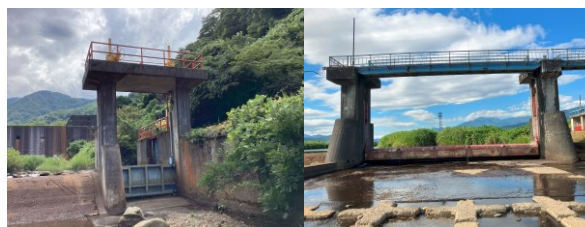
Fig. 1. Tanihama (left) Yashirogawa (right) Headworks.
